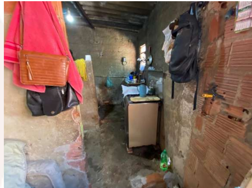
2. Improved kitchen setup with unfinished walls and no ventilation.
